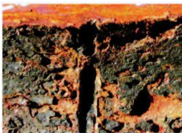
Figure I.21: Severe corrosion at the weldment (deep groove along the weld) indicating that weld metal preferentially corrodes in CO 2 environment
